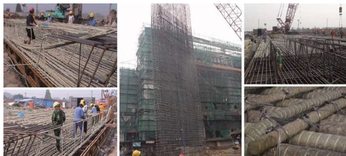
Plate (1-5) GFRP use in the underwater tunnel of Weisan road in Nanjing, China, 2016.
