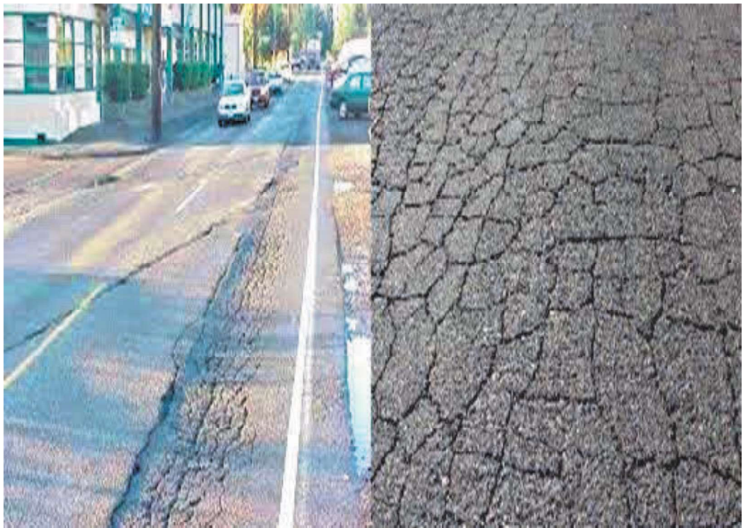
Plate 1.1 Failure of flexible pavement due to weak underlying soils ( www.dailycivil.com )
