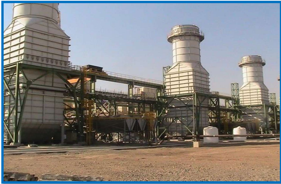
Plate (1.1): Al-Mansuryia power plant station-Diyala/Iraq
