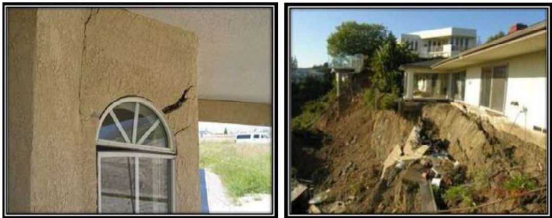
Plate (1.2) Failure of Buildings That are Built on Gypseous Soil (After Abid-Awn, 2010)
