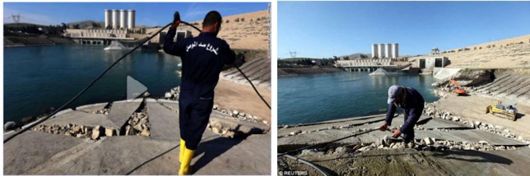
Plate (1.1) Employees Work at Strengthening the Mosul Dam in Northern of Iraq Due to Failure of Gypseous Soil under Construction (Internet source, Alghad Press,2016).
