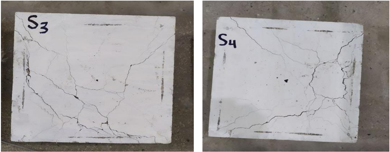
Figure 8. The tested slabs' crack pattern and mode of failure group 1
