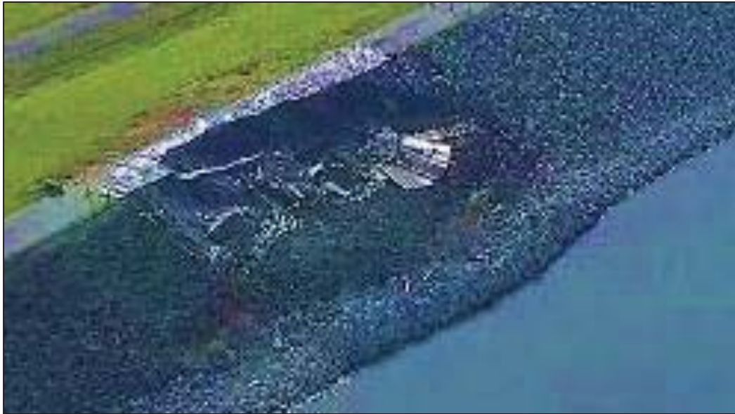
Figure 1.2 Failure of the upstream slope for Salma earth dam(Hamid,2002)
