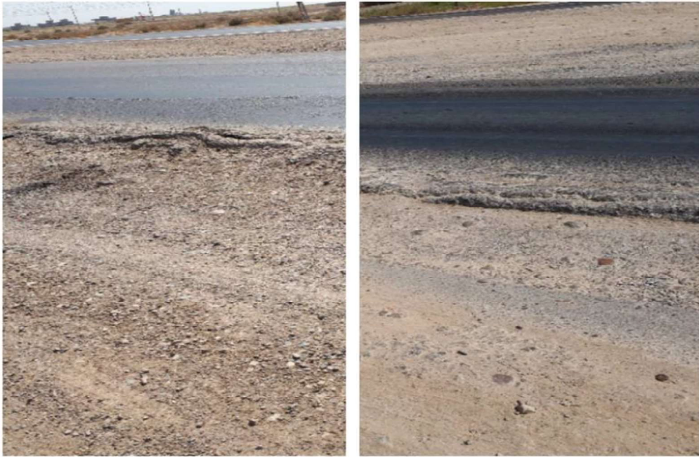
Plate (1.1) Examples of failures of pavements along with Diyala governorates that this study tries to solve geotechnically
