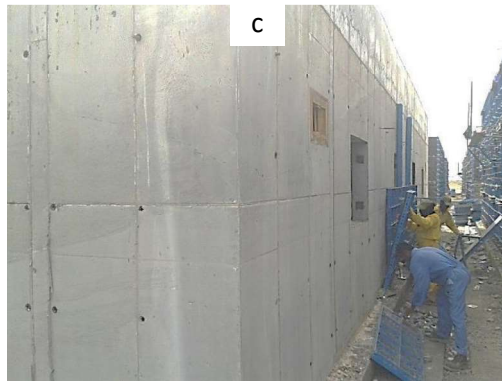
Plate (1-2): (a) Details related to foundations, (b) Installation of molds and casting, (c) Remove the molds after 20 days
