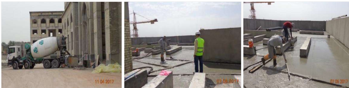
Plate (1-3): The use of LWFC in Al Hussain Quran School in Karbala city, Iraq, 2017.
