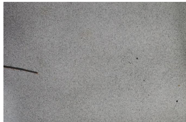
Figure 10. Crack/defect the area
