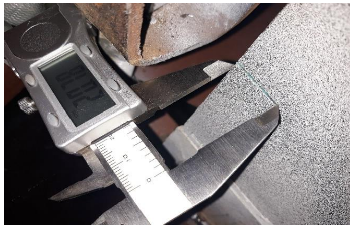
Figure 2. Actual physical crack measurements
