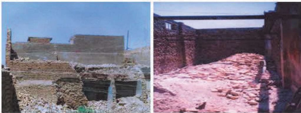
Figure(1-5) Collapse of main walls and roof masonry house in AL Rafee, Iraq in 2004)( ISN,2004).
