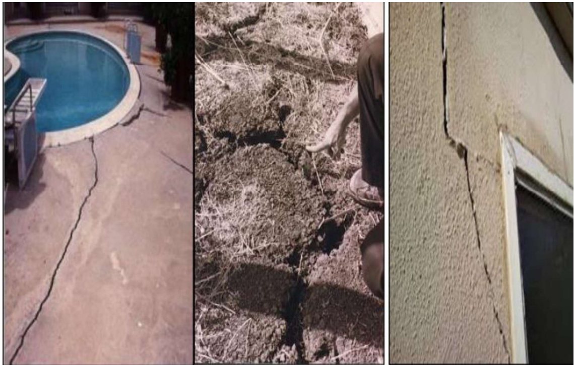
Figure 1.2: The damage of structures and cracks in expansive soil ( Abbas,2016 ).
